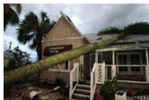
A Royal Palm tree collapsed into this Landmark Realty office building in Punta Gorda.
