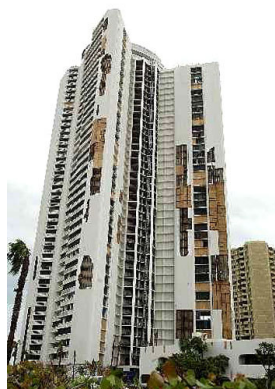
The Tiara, a large high-rise condominium complex on Singer Island, received damage from hurricane Jeanne. The building had also been damaged from hurricane Frances.
